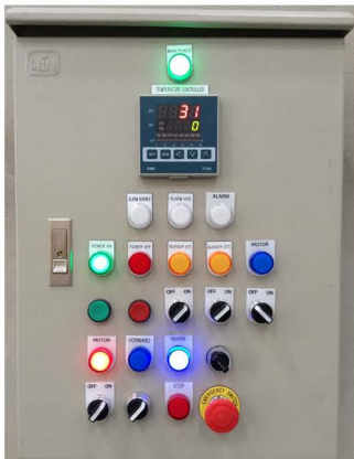
Digital Controller Panel burner
