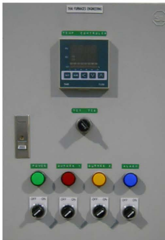
Digital Controller Panel burner
